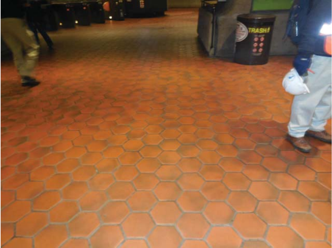
Pictures 1&2: K02 Clarendon – No handholes in mezzanine
