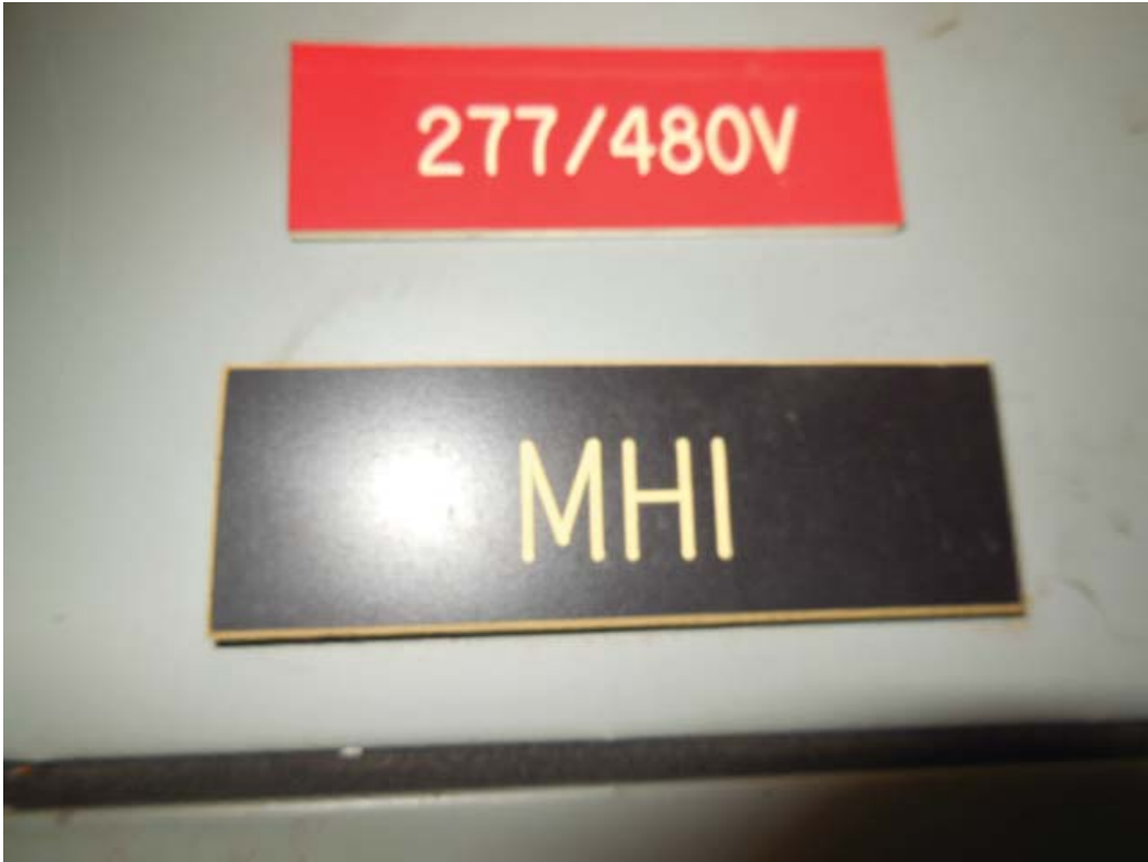
Pictures 16&17: K06 West Falls Church – Panels MHI & ML2 into common trough in Room 212
