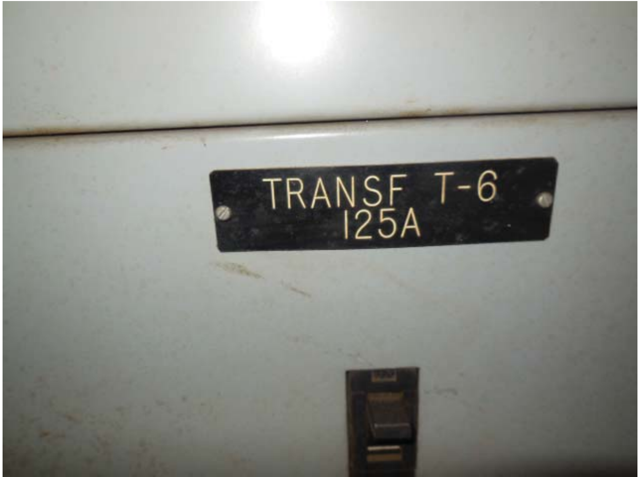
Picture 13 K08 Vienna – TRANSF T-6 125A in Room 106
