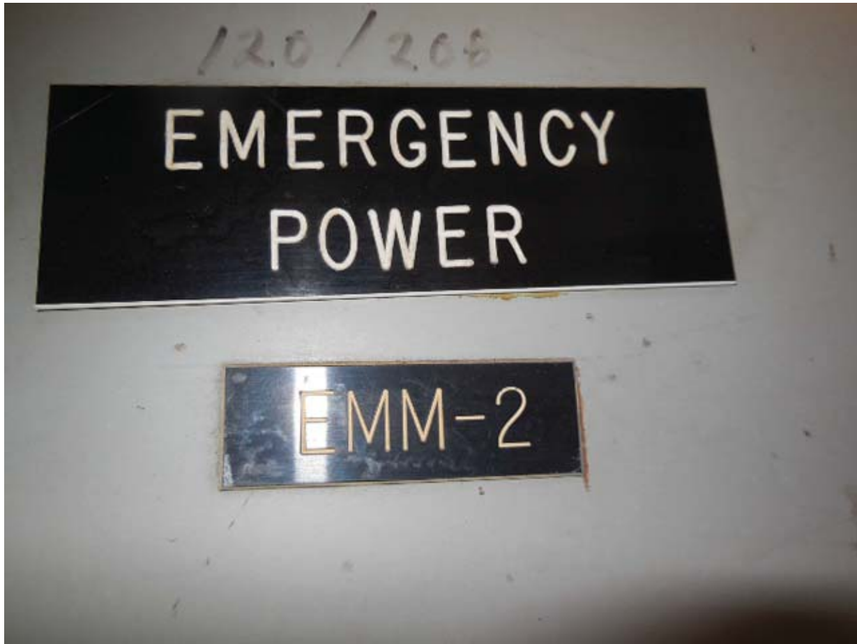
Picture 3: K07 Dunn Loring – Emergency panel EMM-2 in Room 301
