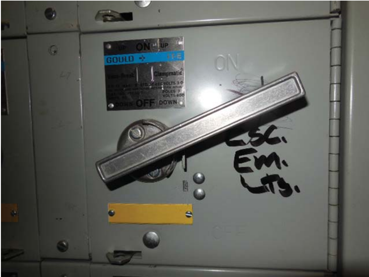
Pictures 4: K07 Dunn Loring – Emergency panel EMM-2 in Room 301 - Breaker 4
