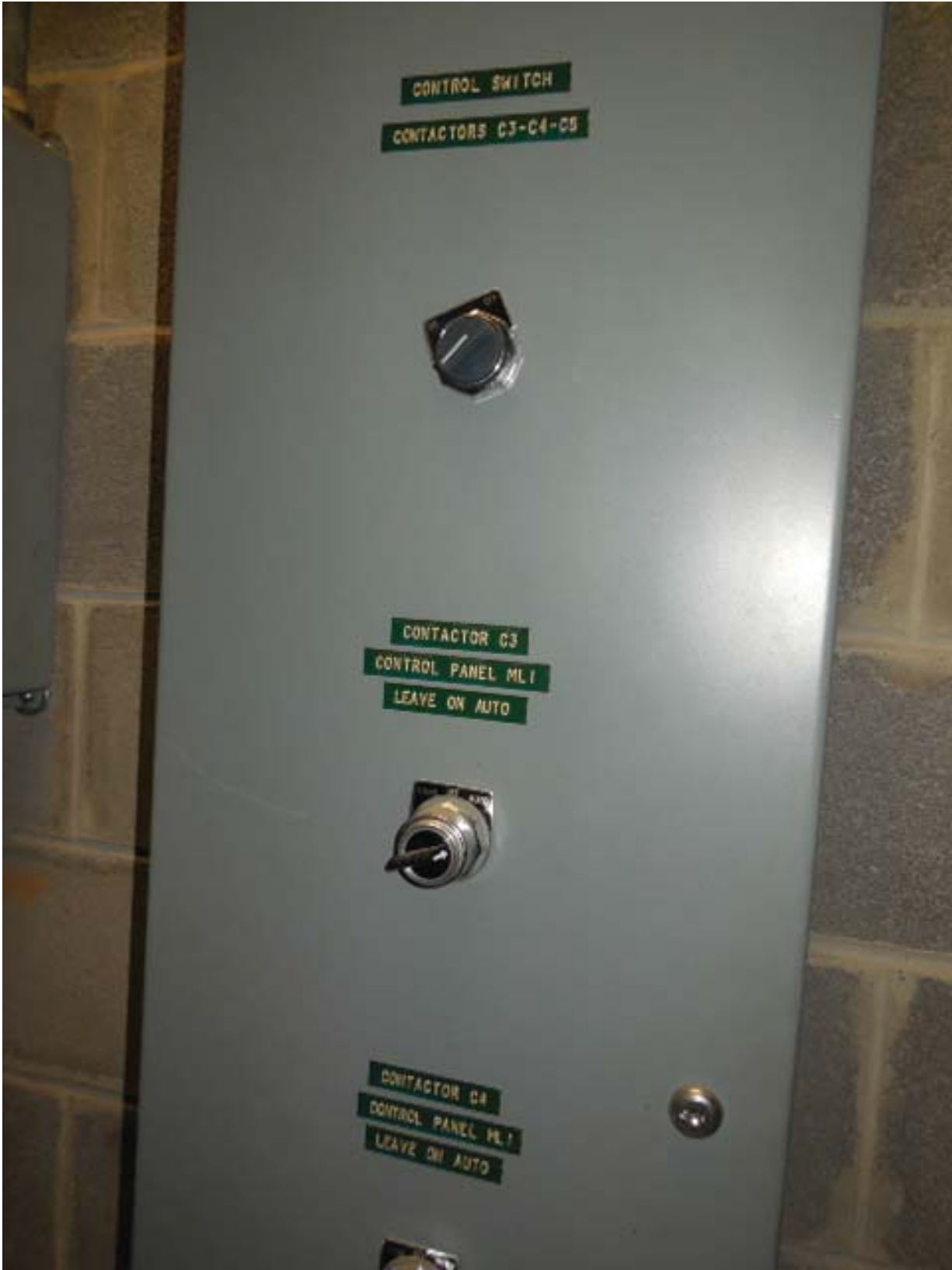
Picture 15: K06 West Falls Church – Control switch panel into common trough in Room 212
