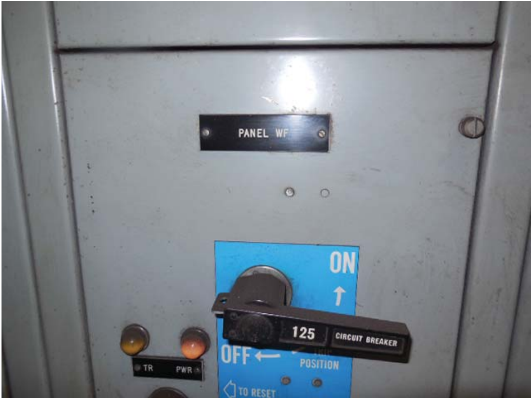
Picture 14: K03 Virginia Square-GMU – West Essential Power SWBD in room 104, Panel WF breaker
