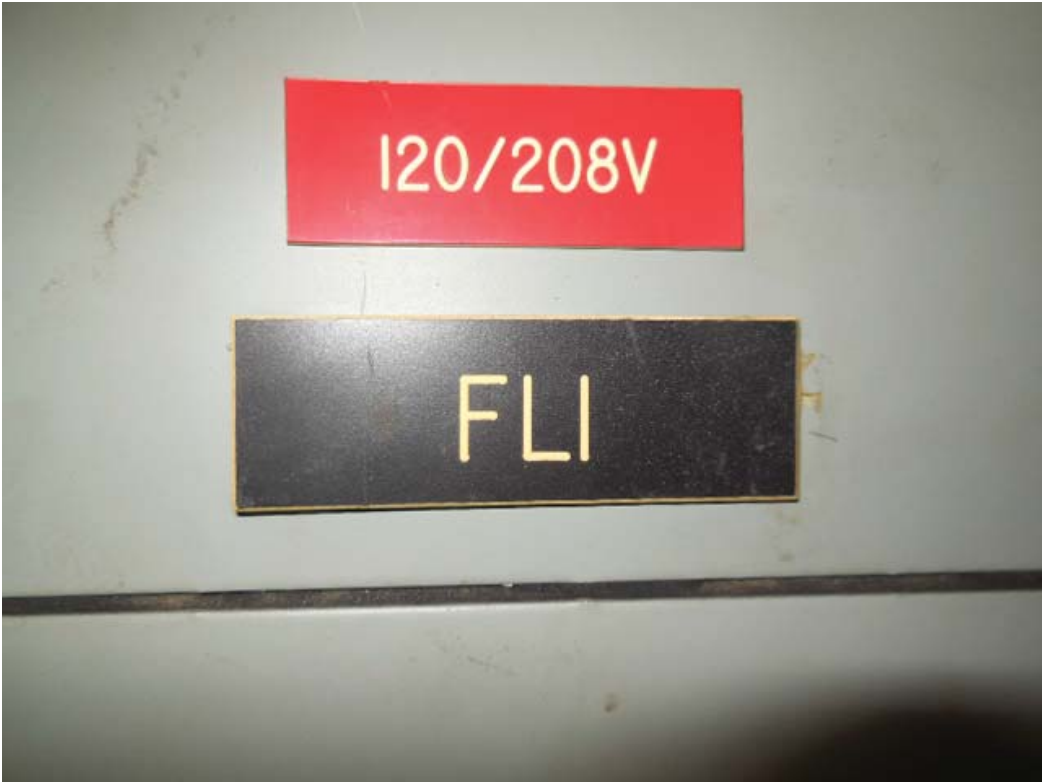
Pictures 9&10: K06 West Falls Church – AFC Panel FL-1 & bottom of panel in Room 212
