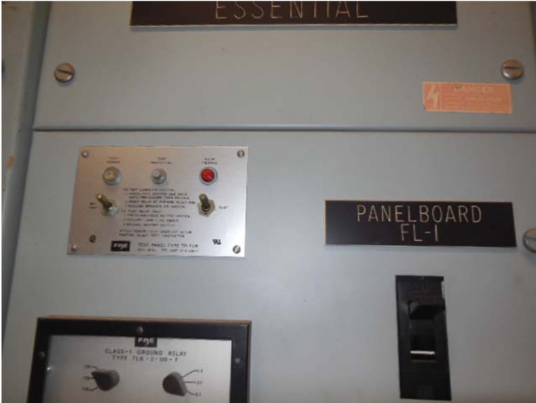
Pictures 24&25: K06 West Falls Church – Panel board breakers FL-1 & MH-1 in Room 106
