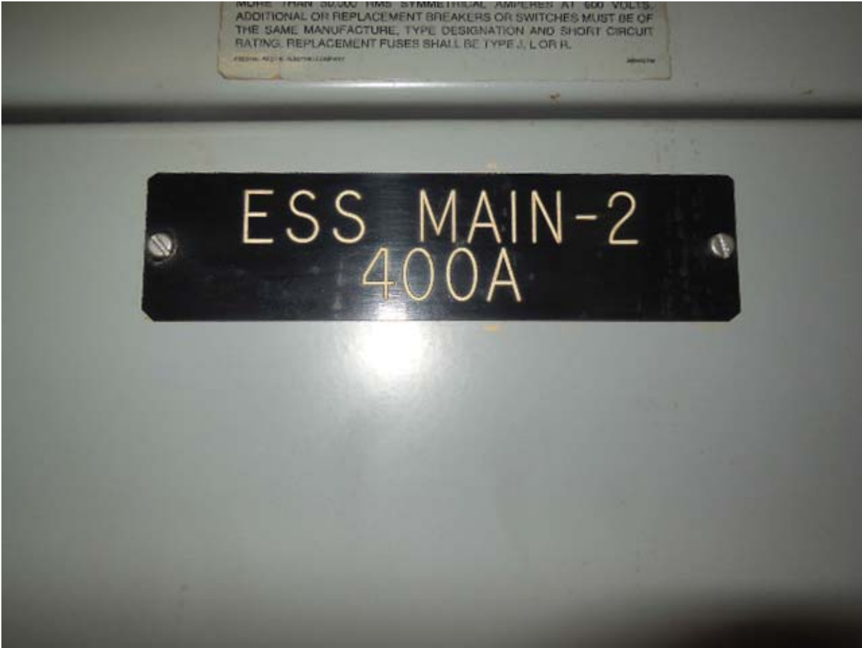
Picture 12 K08 Vienna – ESS Main-2 400A in Room 106
