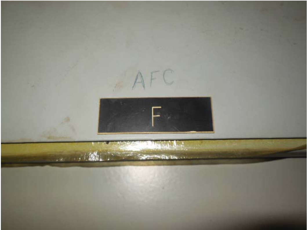
Picture 6: K05 East Falls Church – AFC Panel F in room 115
