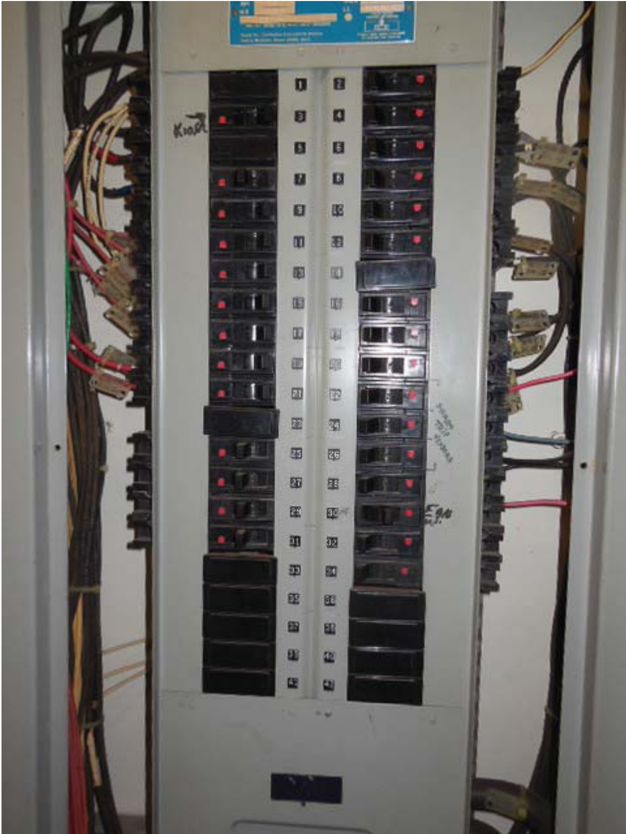
Picture 6: K07 Dunn Loring – AFC Panel ESF-1 in Room 301
