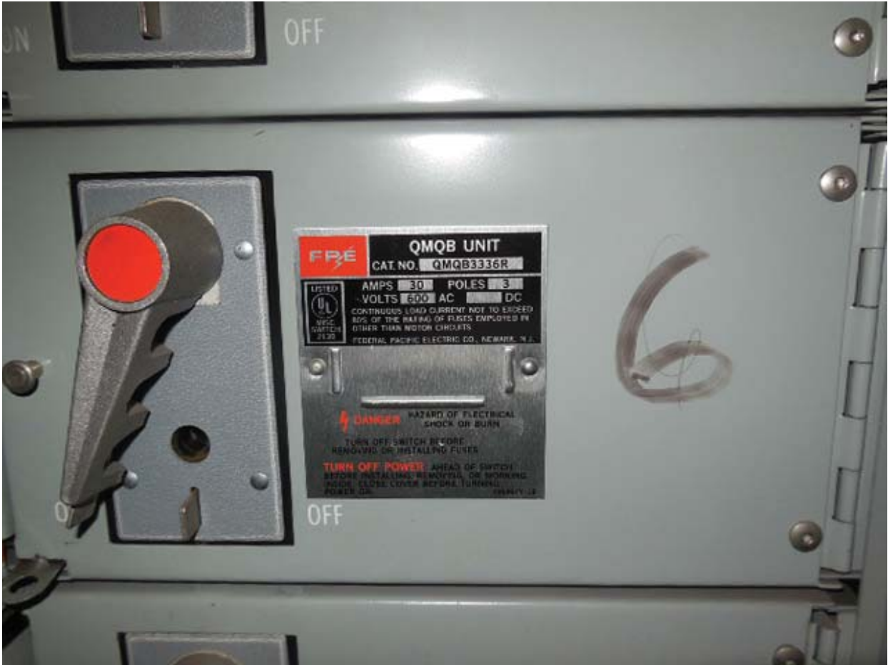
Pictures 4: K08 Vienna – Emergency panel ELIVI in Room 202 - Breaker 6
