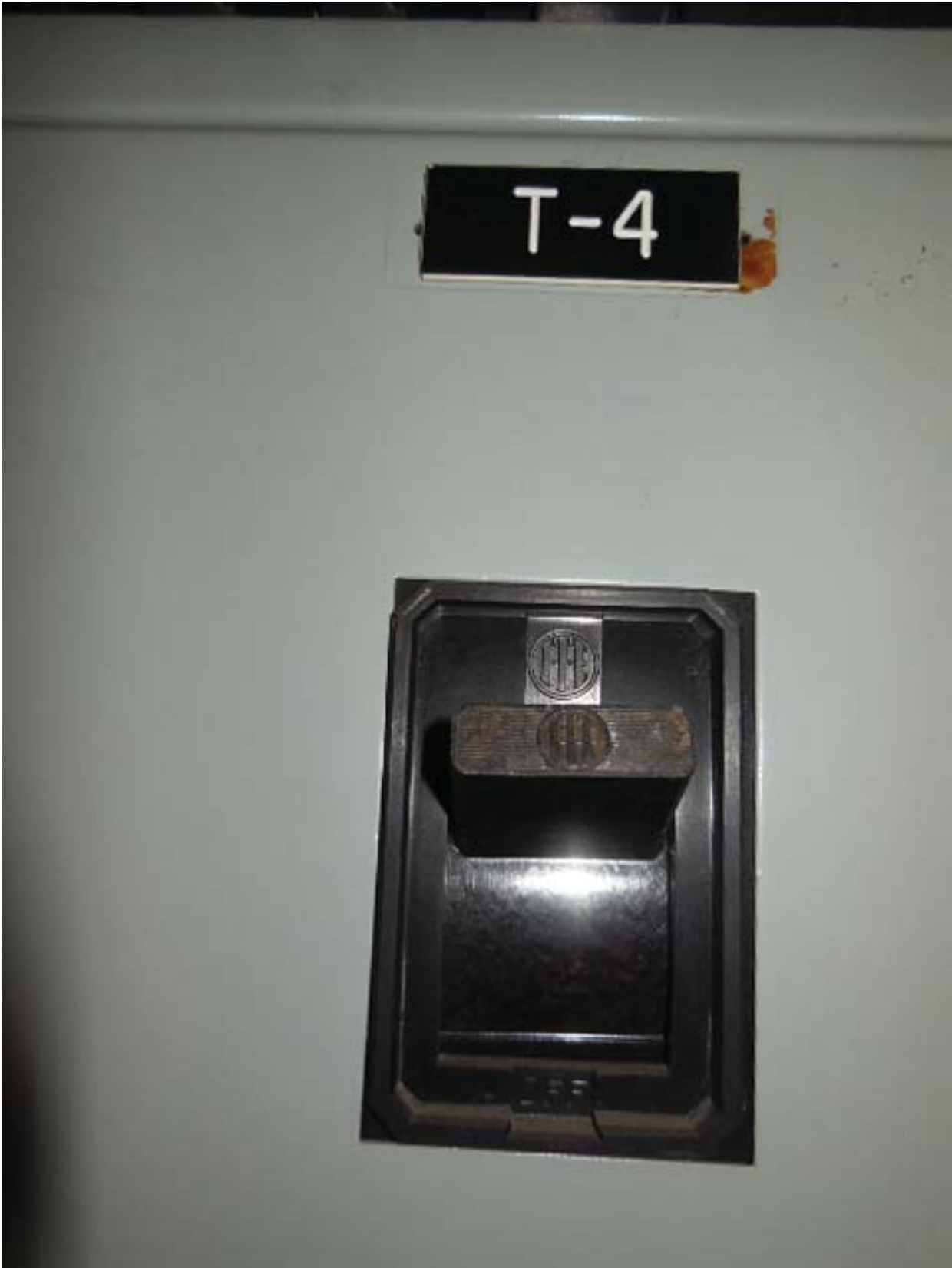
Picture 9: K07 Dunn Loring – AFC source breaker 'T-4' in Room 111
