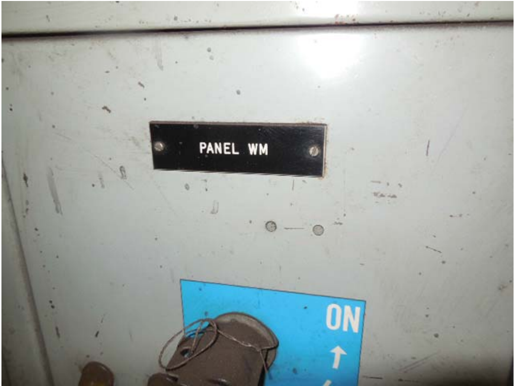
Picture 15: K03 Virginia Square-GMU – West Essential Power SWBD in room 104, Panel WM breaker
