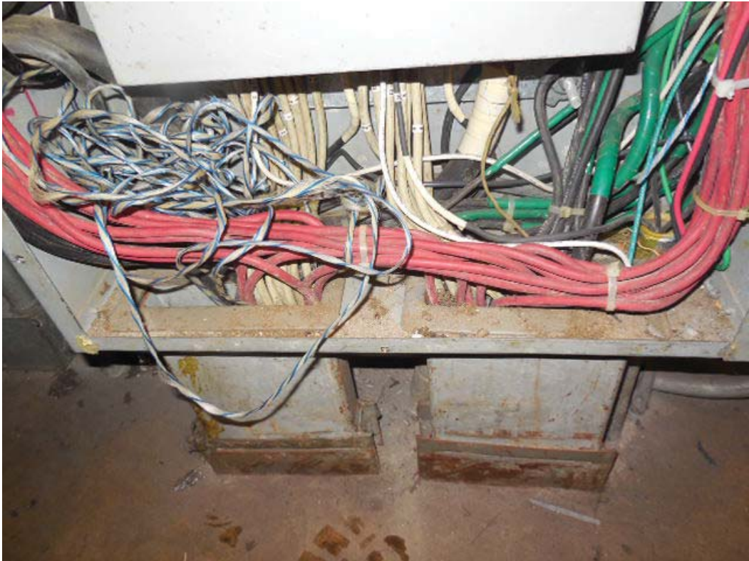
Picture 8: K05 East Falls Church – AFC Panel F in room 115, Bottom ducts
