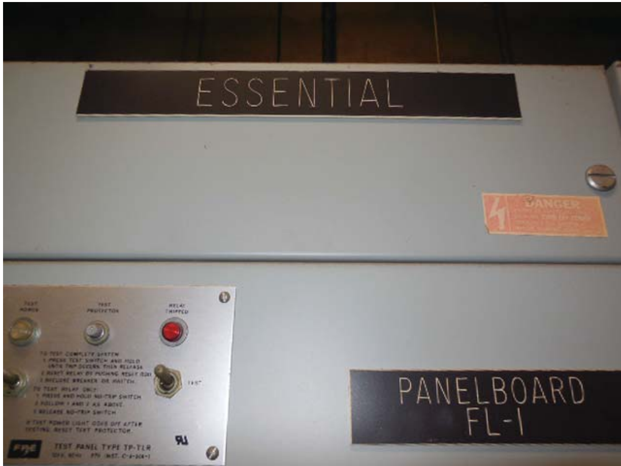
Picture 23: K06 West Falls Church – Essential switchboard in Room 106
