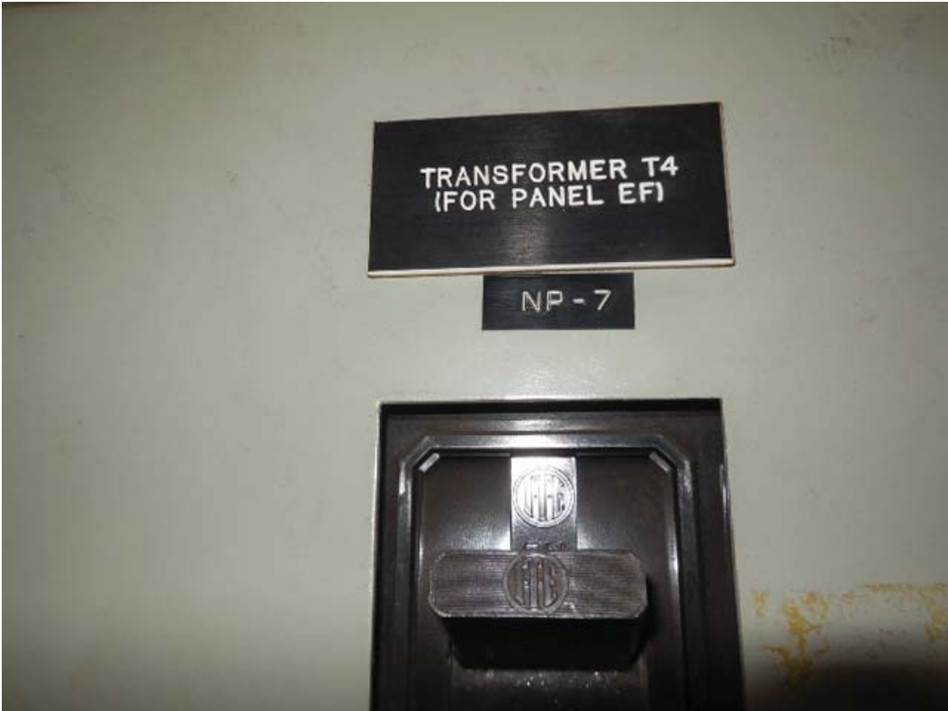
Picture 4: K01 Court House – Transformer T4 breaker (NP-7) for Panel EF in room 305
