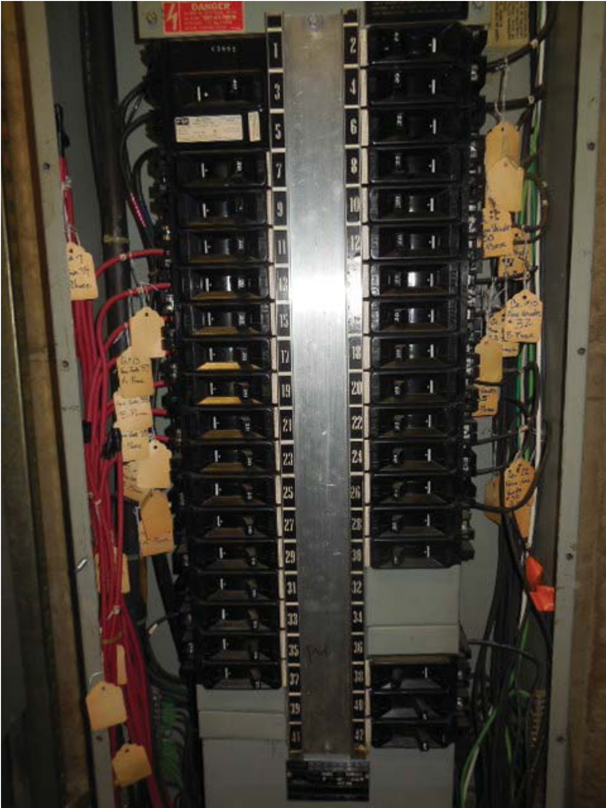
Picture 11: K06 West Falls Church – AFC Panel FL-1 in Room 212
