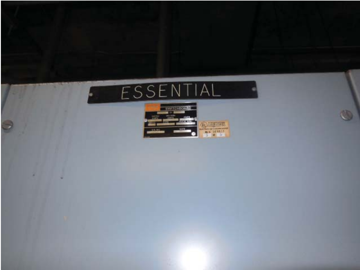
Picture 11 K08 Vienna – Essential SWBD in Room 106
