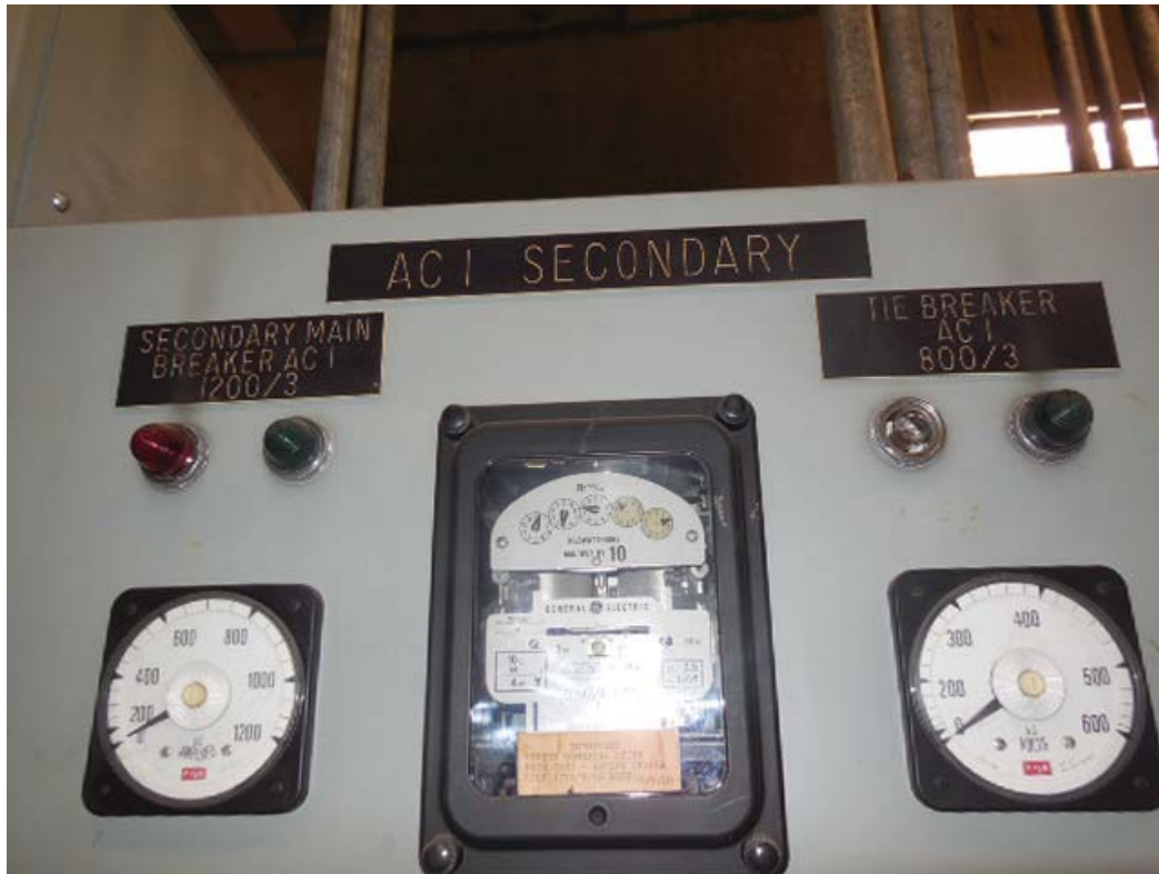
Pictures 10&11: K05 East Falls Church – AC1 Secondary SWBD & breaker #7 for Panel F in room 116
