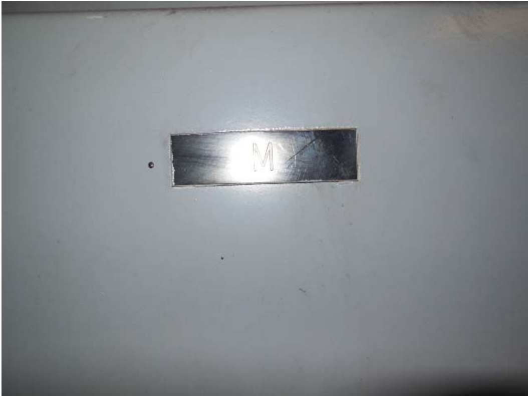
Picture 9: K02 Clarendon – AFC Panel M in room C203
