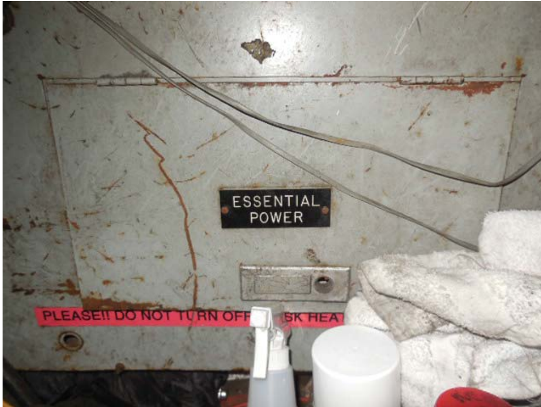
Pictures 4&5: K05 East Falls Church – Emergency Panel KE in Kiosk
