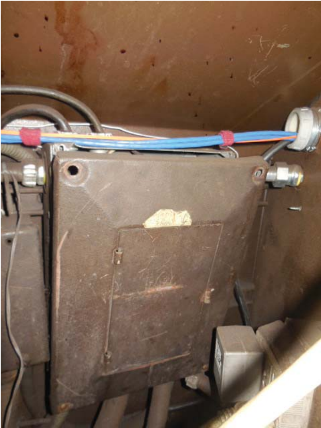
Picture 4: K02 Clarendon – Emergency Panel KE in Kiosk
