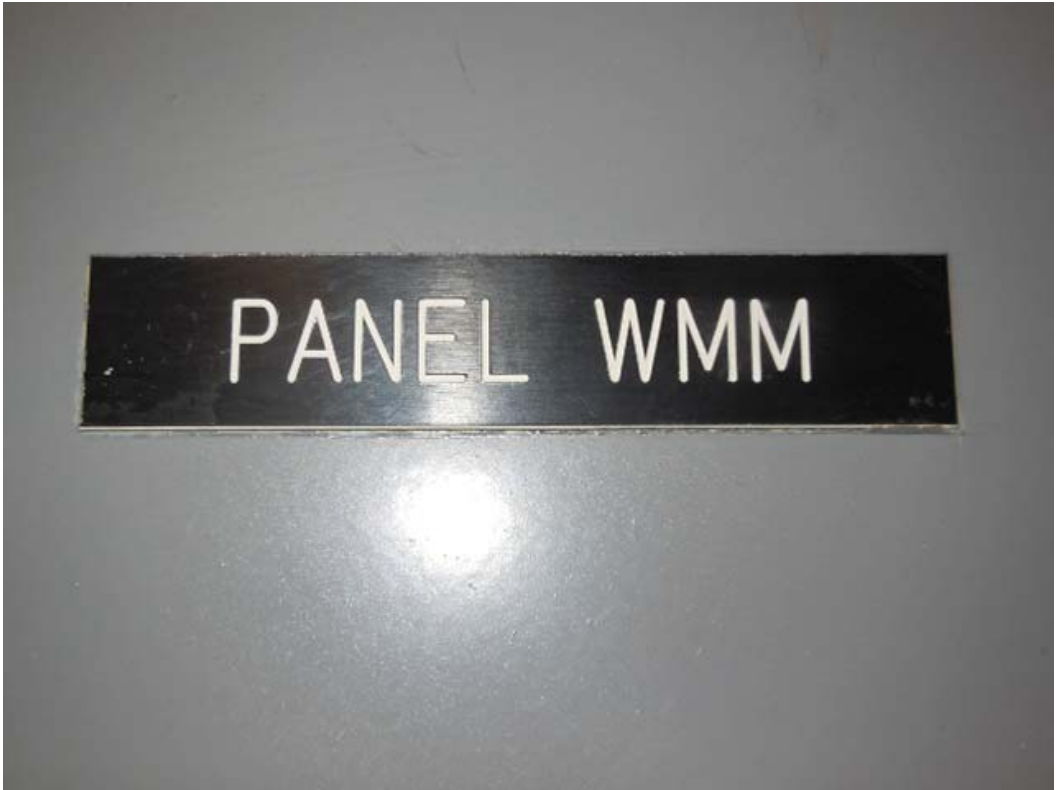
Pictures 22&23: K03 Virginia Square-GMU – Panels WMM & WPOB in room C206
