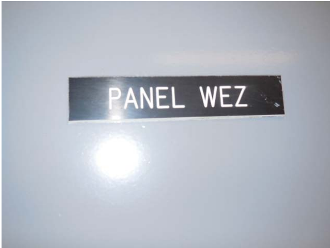
Pictures 18&19: K03 Virginia Square-GMU – Panel WEZ & panel schedule in room C206
