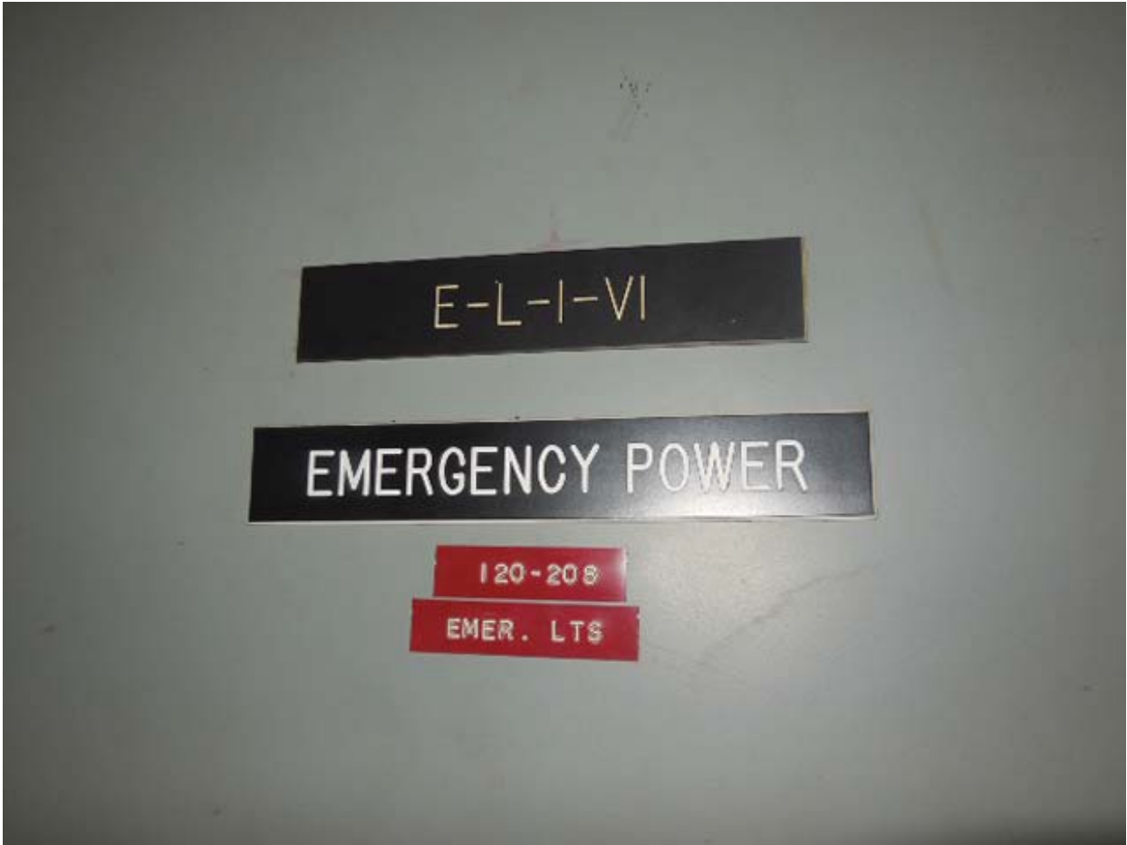
Picture 3: K08 Vienna – Emergency panel ELIVI in Room 202
