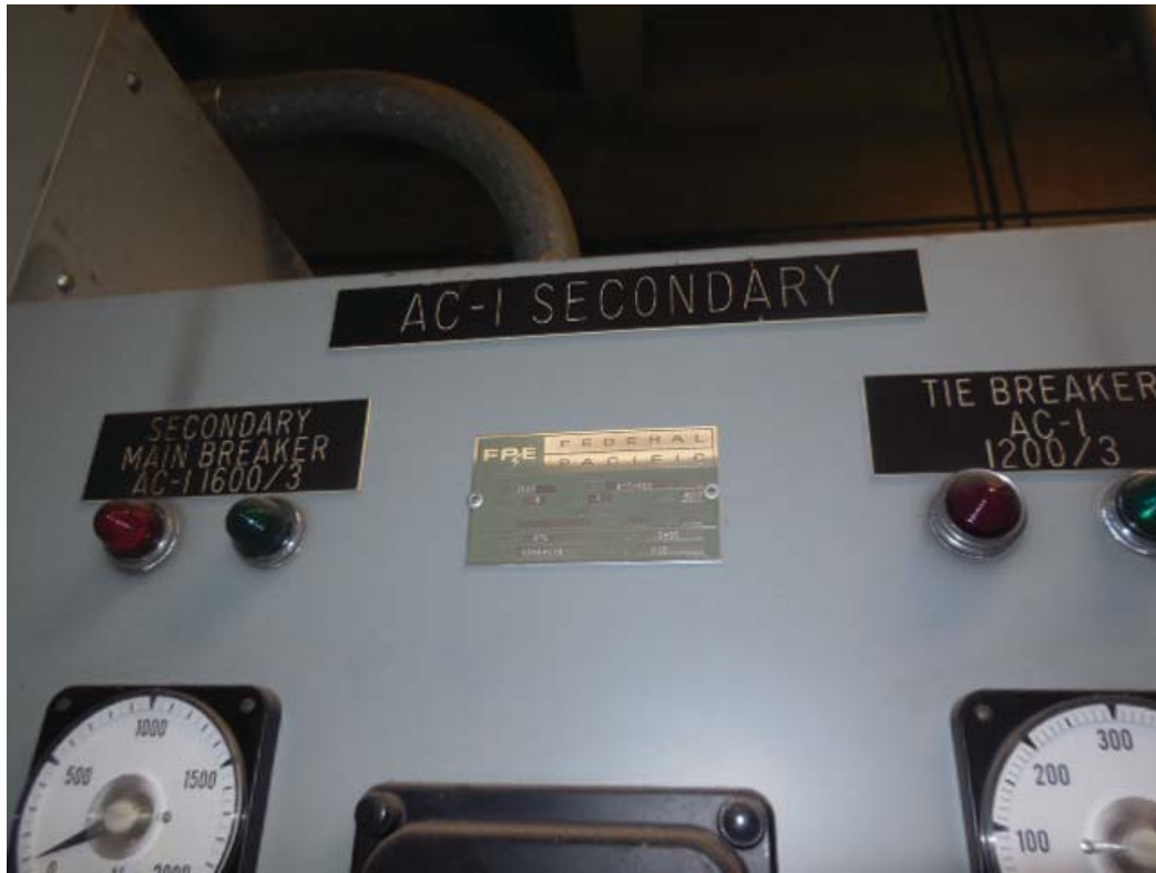
Pictures 21&22: K06 West Falls Church – Switchboards AC-1 Secondary & AC-2 Secondary in Room 106
