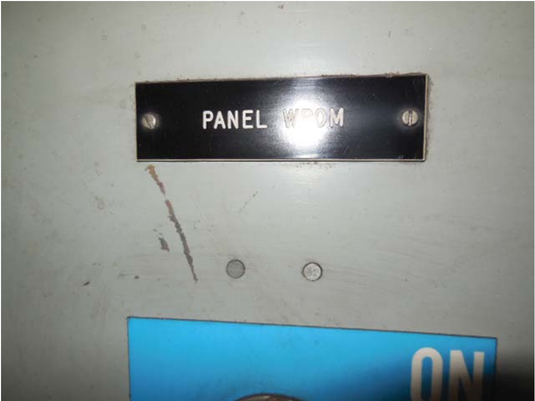
Picture 17: K03 Virginia Square-GMU – West Non-essential Power SWBD in room 104, Panel WPOM BRK
