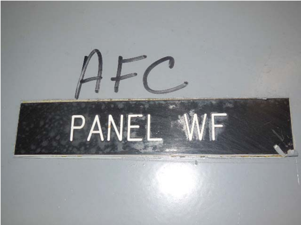
Picture 5: K03 Virginia Square-GMU – AFC Panel WF in room C206
