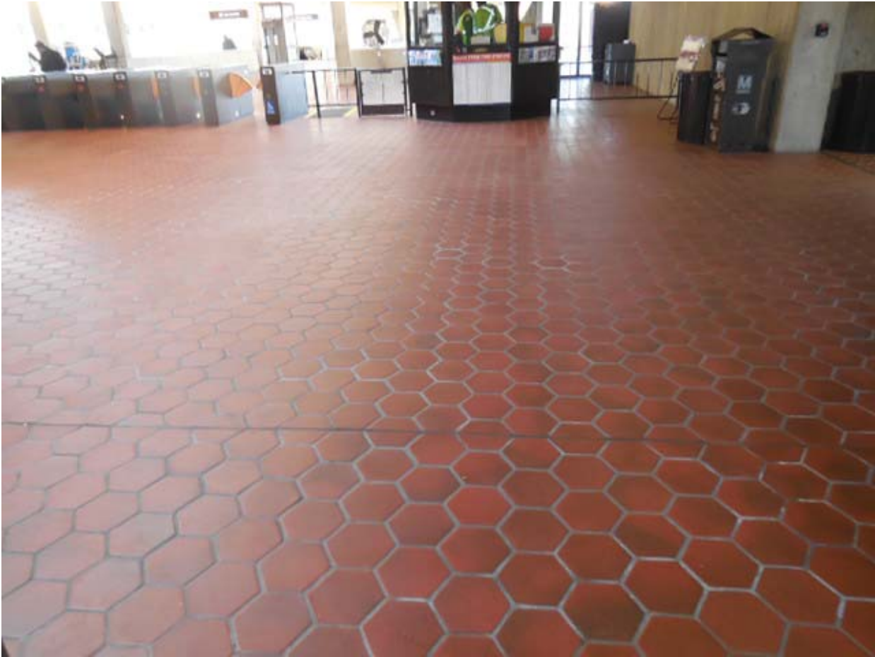
Picture 1: K06 West Falls Church – No handholes in Mezzanine
