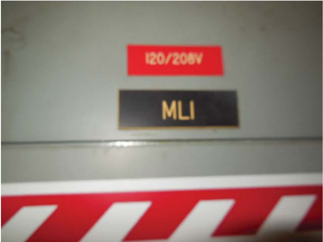
Pictures 18&19: K06 West Falls Church – Panels MLI & MMLI into common trough in Room 212
