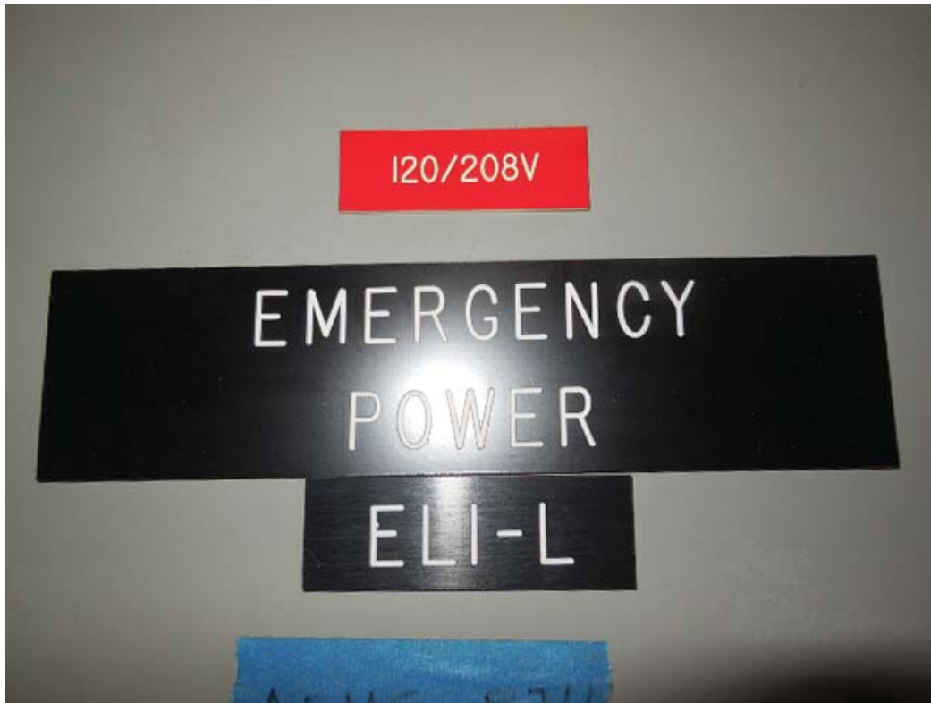
Pictures 6&7: K06 West Falls Church – Emergency power panel ELI-L & breaker 16 in Room 106
