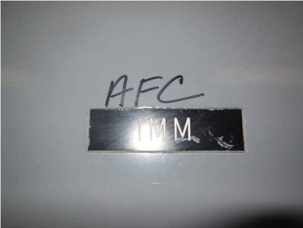
Picture 5: K02 Clarendon – AFC Panel IMM in room C203
