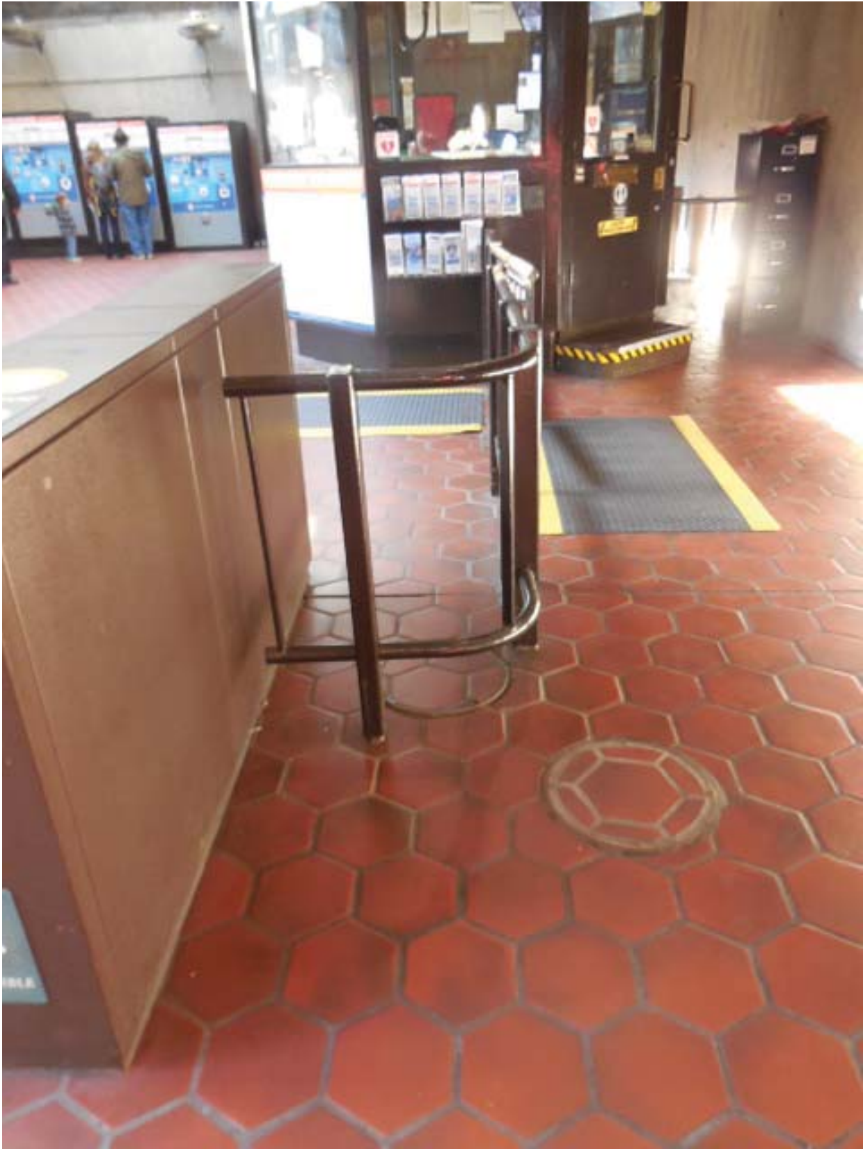
Picture 1: K07 Dunn Loring – Handholes in Mezzanine
