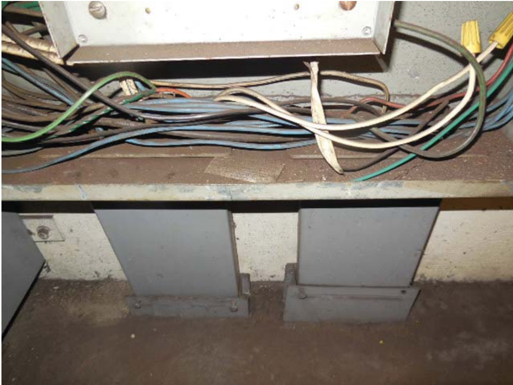
Picture 7: K02 Clarendon – AFC Panel IMM in room C203, Bottom ducts
