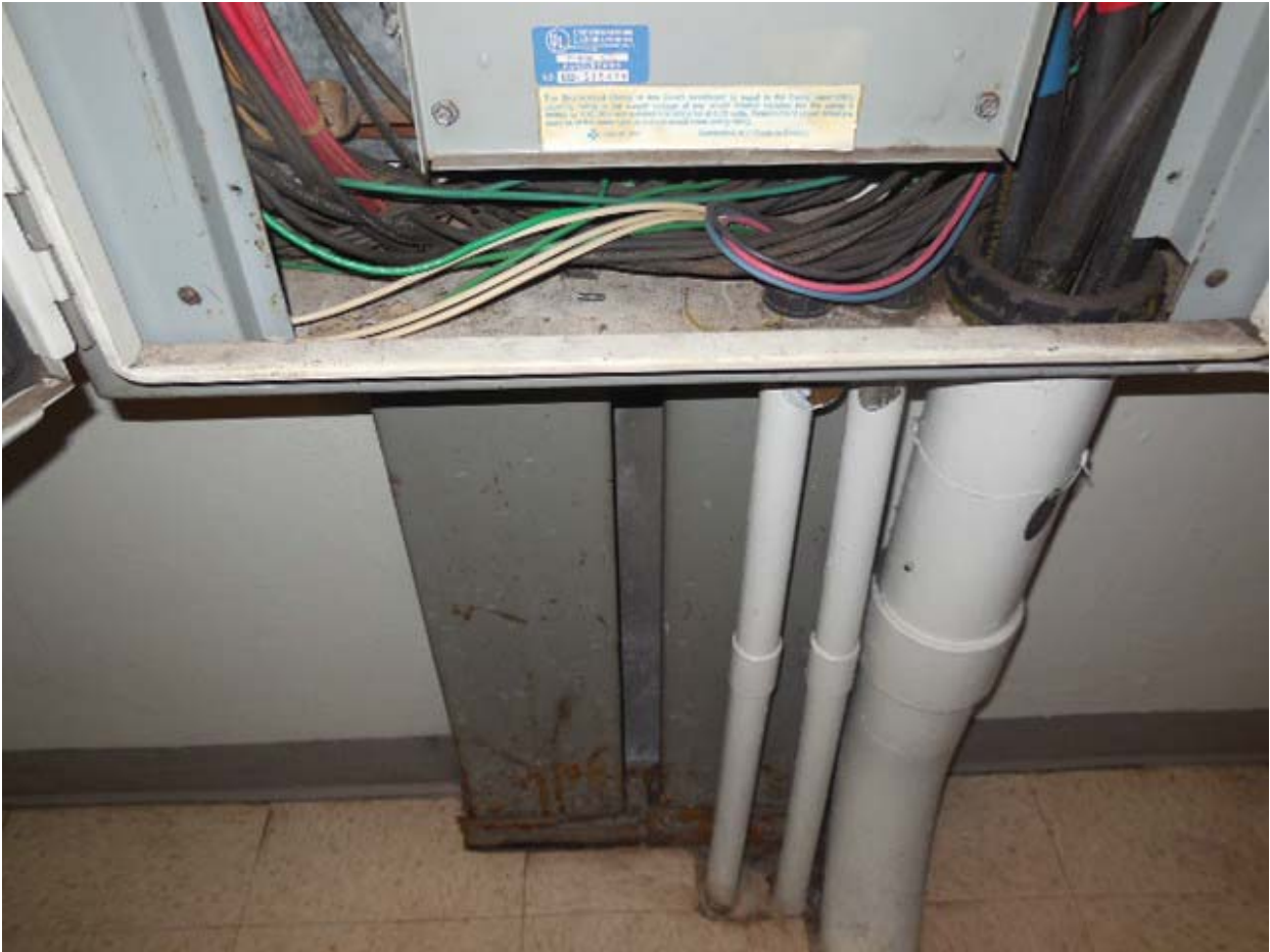
Picture 7: K07 Dunn Loring – AFC Panel ESF-1 in Room 301 – Bottom duct and conduits
