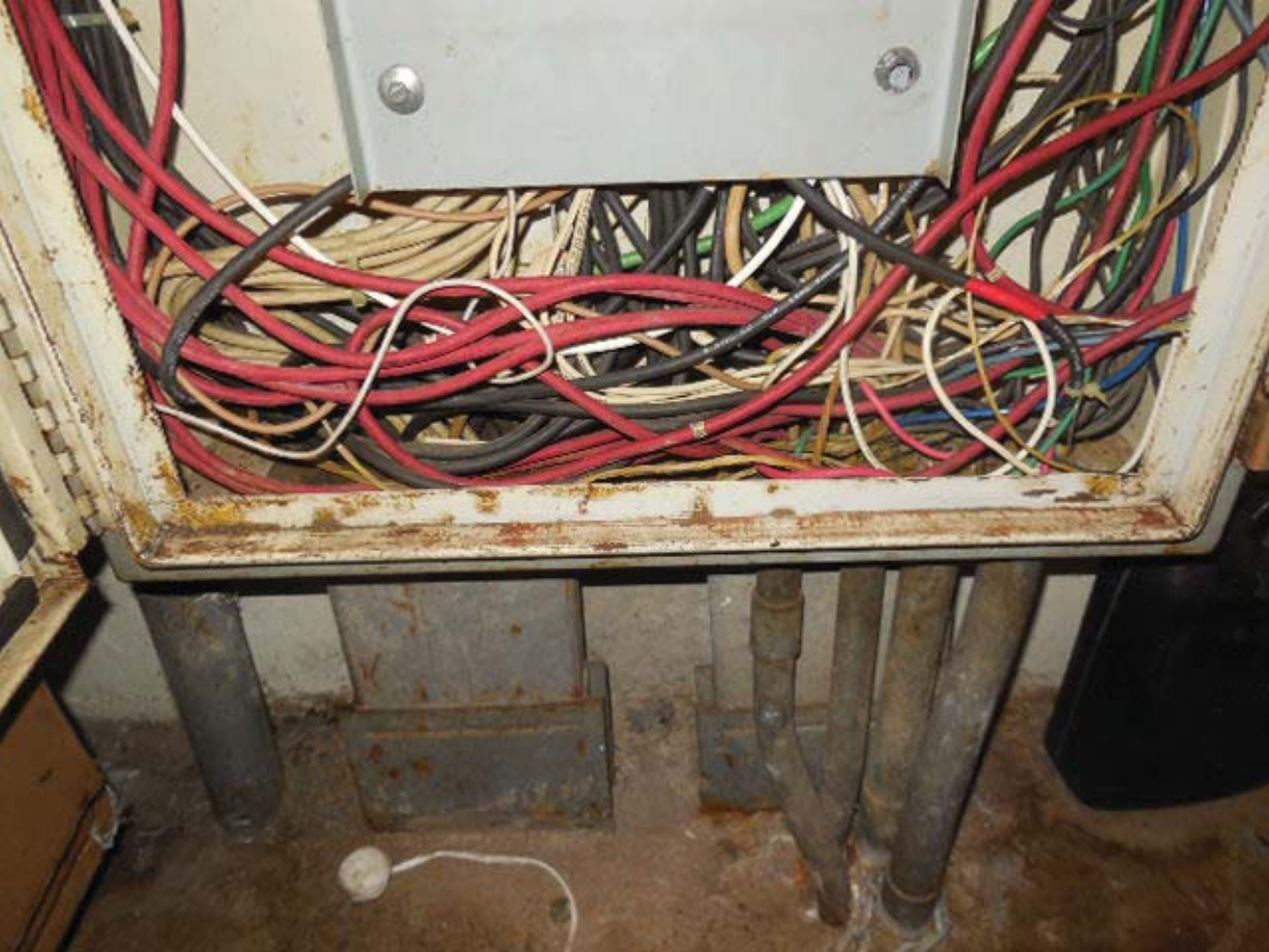
Picture 9: K08 Vienna – AFC Panel ESLFMV in Room 406 – Bottom duct and conduits
