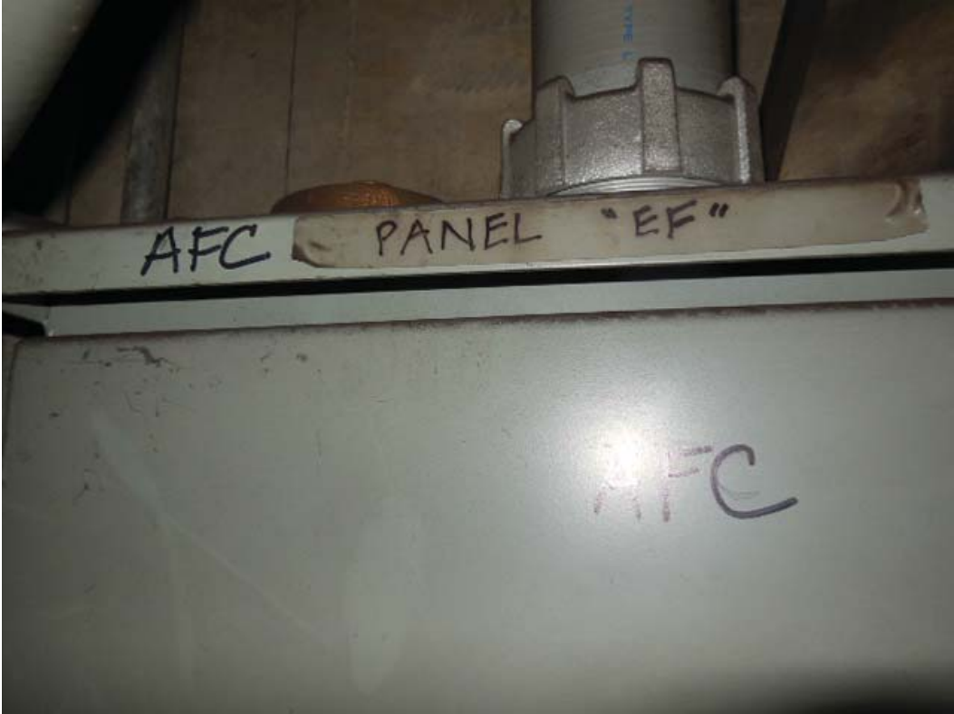
Picture 5: K01 Court House – AFC Panel EF in room 205
