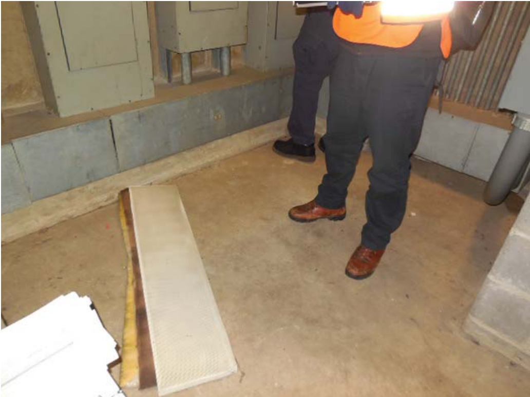
Pictures 13&14: K06 West Falls Church – Common trough in Room 212
