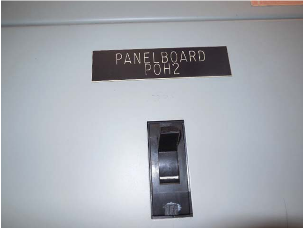
Picture 26: K06 West Falls Church – Panel board breaker POH2 in Room 106
