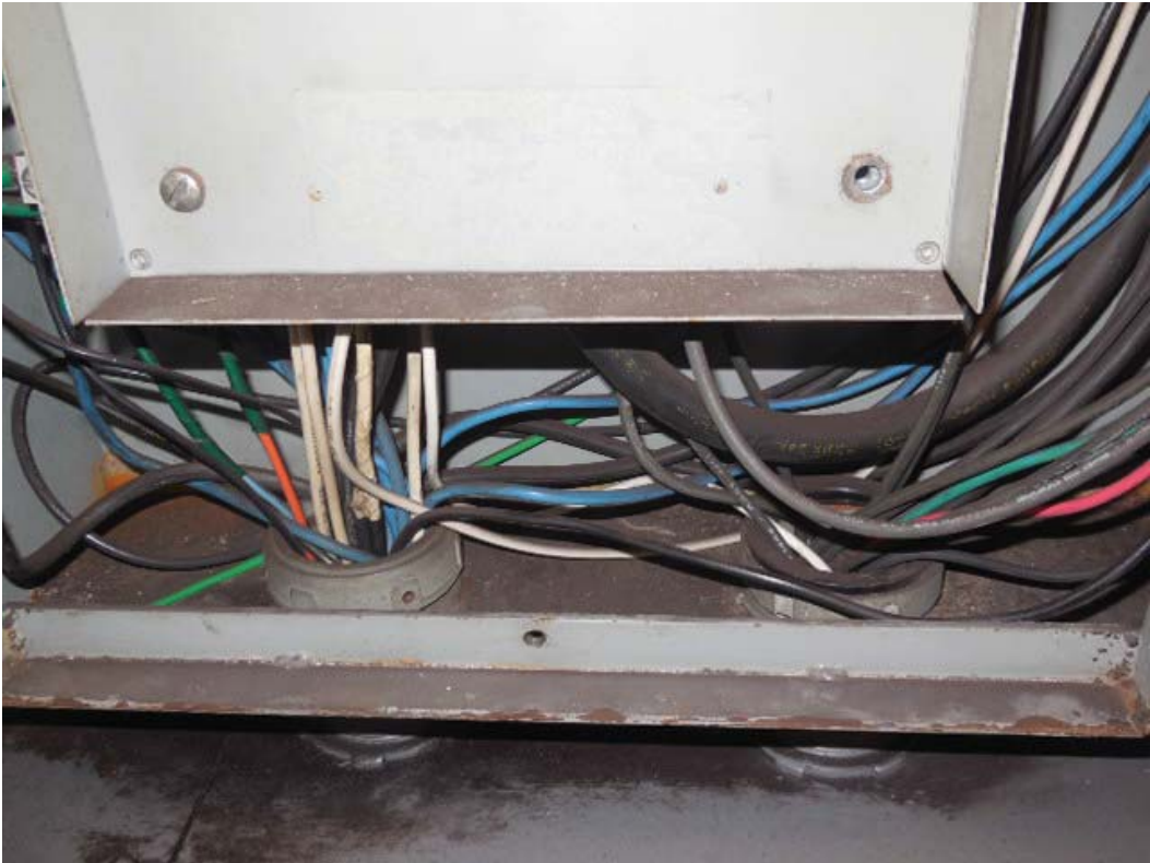
Picture 7: K03 Virginia Square-GMU – AFC Panel WF in room C206, bottom conduits
