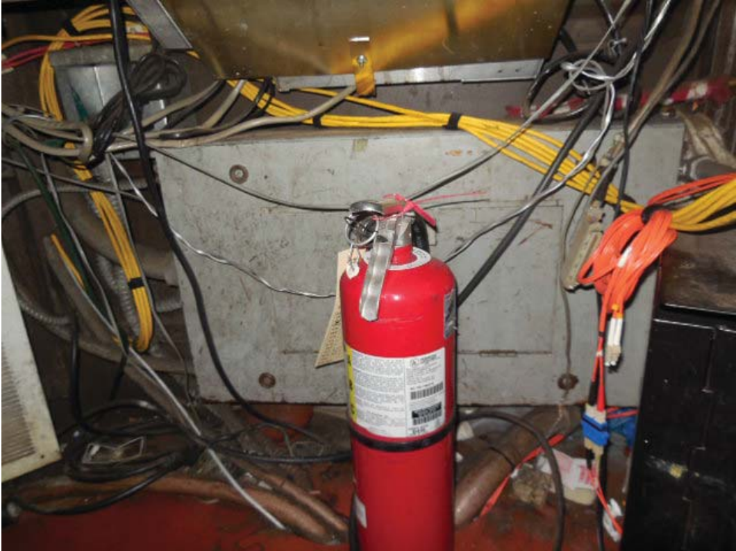
Pictures 4&5: K06 West Falls Church – Emergency panels in Kiosk
