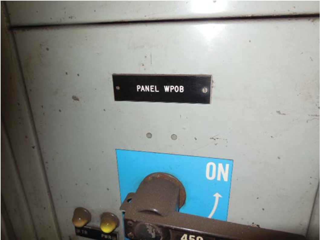
Picture 16: K03 Virginia Square-GMU – West Essential Power SWBD in room 104, Panel WPOB breaker
